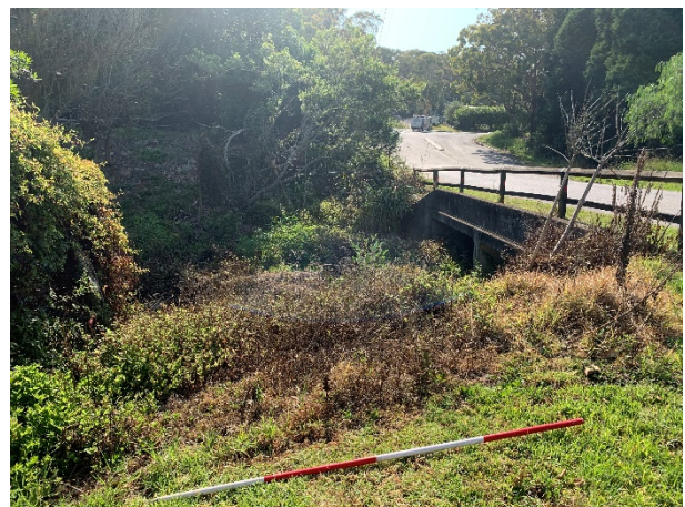
Plate 14: View showing the concrete bridge located to the south of the school site where Dreadnought Road crosses the stream.
